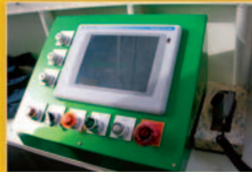
X Scream controls with PanelView Plus operator interface.
